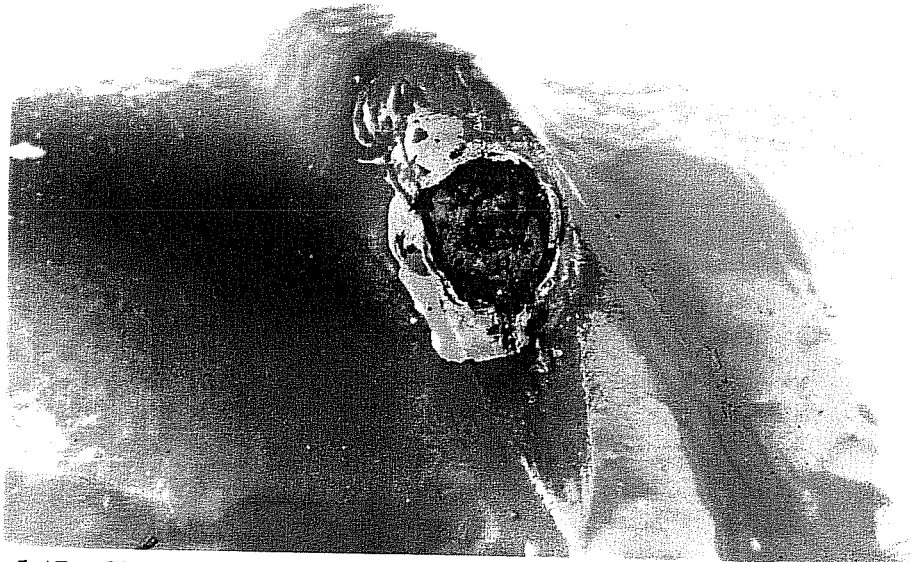
Photo 5.47. Close-up picture of a broken blister showing the corrosion products accumulated within it.
