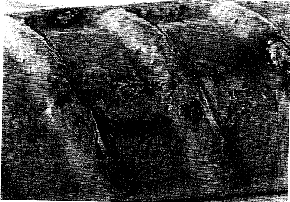
Photo 5.44. Another close-up picture also showing cracks formed on ECR after immersion in NaCl solution.
